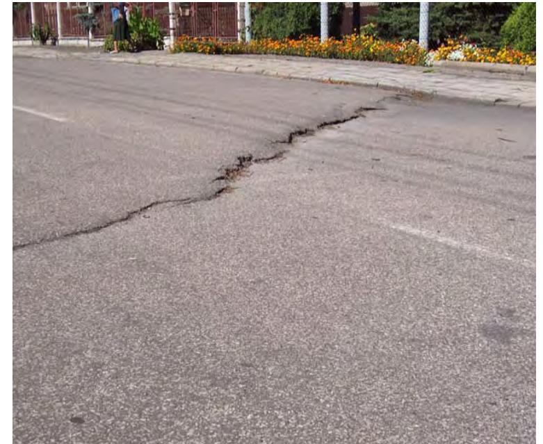
Fig.2 Example of fault occurrence, crosswise the roadway (Strzałkowski, Scigala, 2003)
